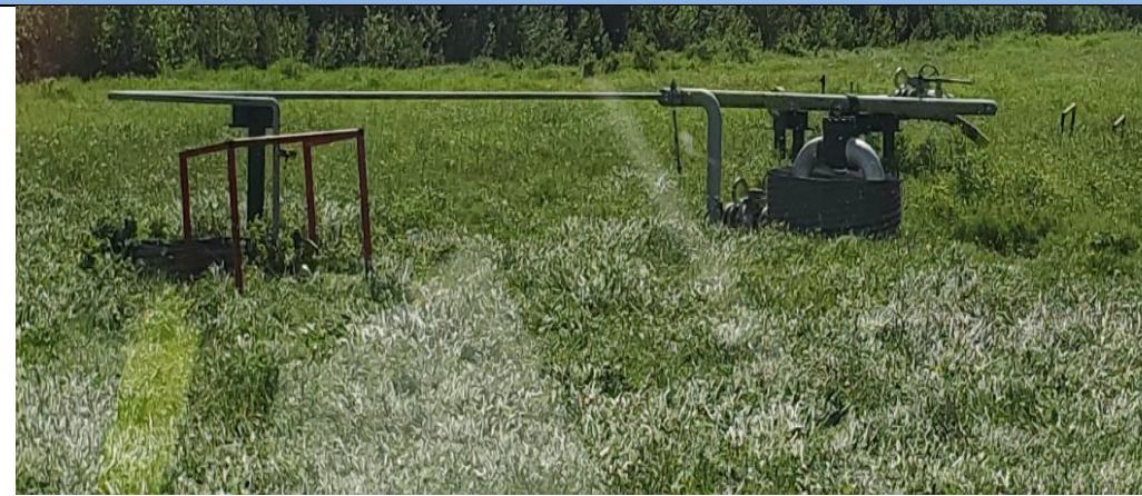
PM-6 Above Ground Bypass Piping
