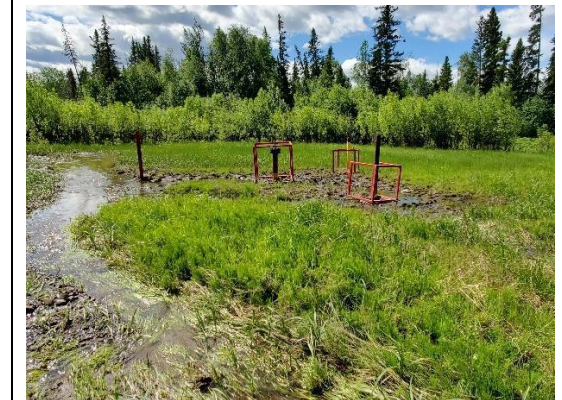
PM-7 Flare Riser and Supports
