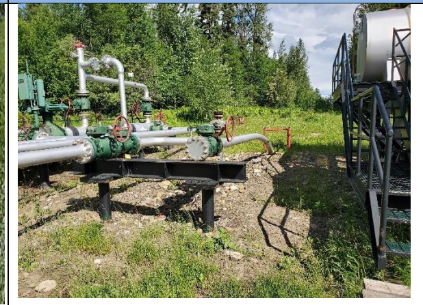
PM-7 Launcher and Bypass Piping
