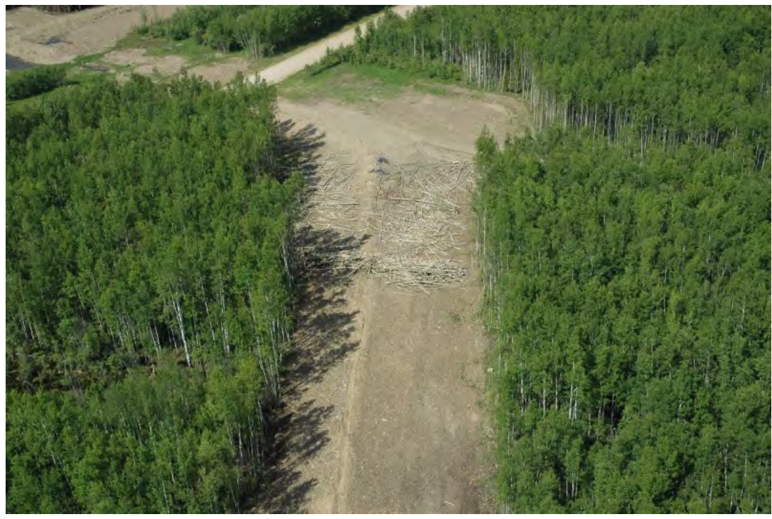
Plate 13 Example of a log berm combined with woody debris rollback for access management and line-of-sight break. The woody debris is placed along the pipeline right-of-way, set back from the wider road crossing area (extra temporary workspace was needed to install the pipeline across the road). By setting back the debris rollback and berm, a larger area of coverage could be achieved than would be possible immediately adjacent to the road. Photo source: CH2M HILL.
