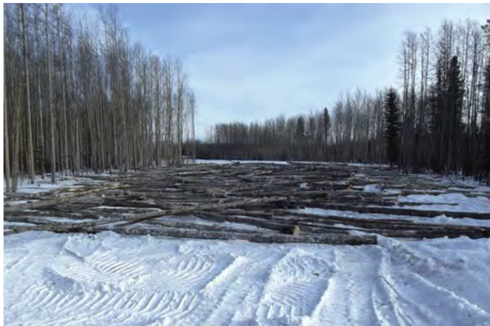
Plate 2: Example of coarse woody debris rollback for access management on a non-parallel pipeline ROW. The debris also creates microsites to enhance vegetation establishment and growth. Photo source: NGTL.
