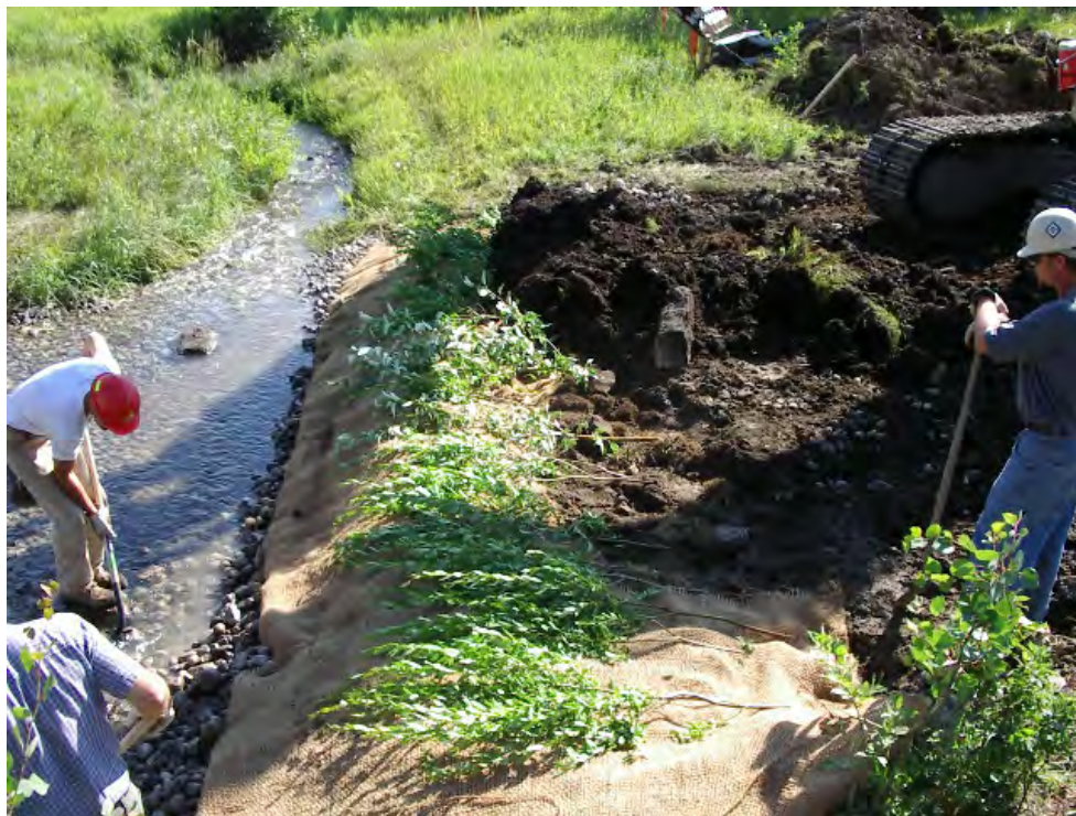
Plate 12: Example of shrub staking in the riparian area at a watercourse crossing. Photo source: NGTL.
