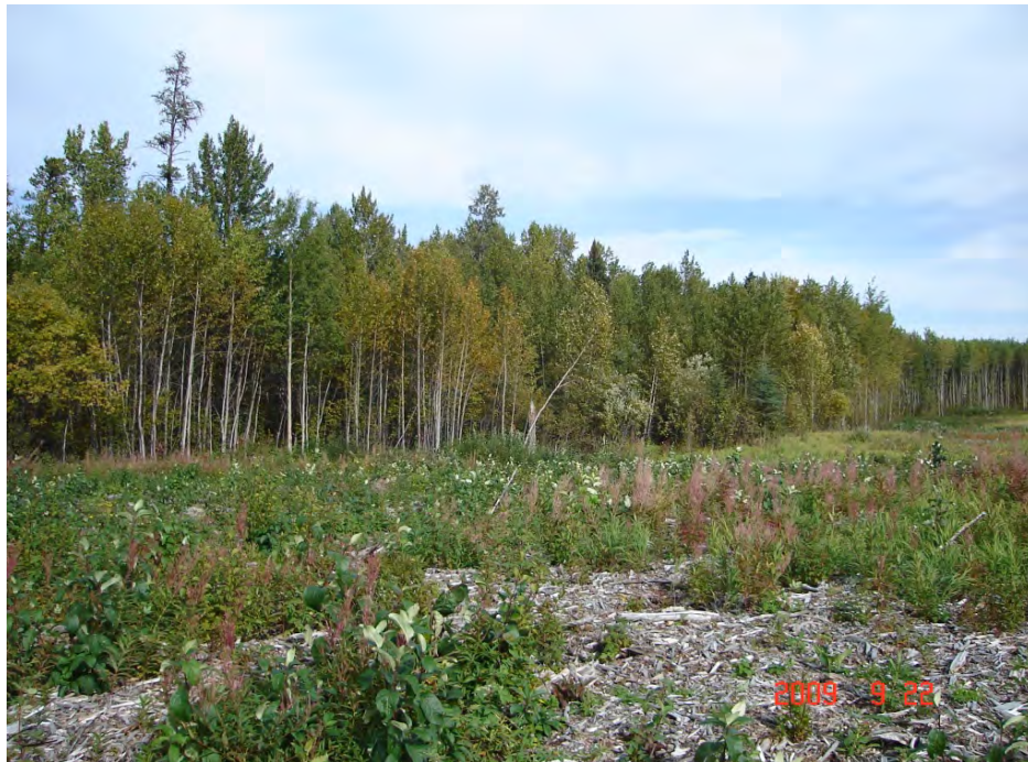
Plate 1: Example of the effectiveness of minimal disturbance construction in forested areas. Photo shows growth after one growing season. Photo source: NGTL.
