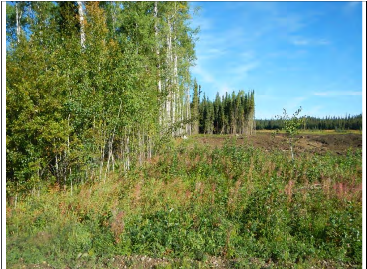
Figure 5 Example of Minimum Disturbance Construction, Hand-Cutting of Vegetation along a Pipeline ROW, at a Road Intersection
