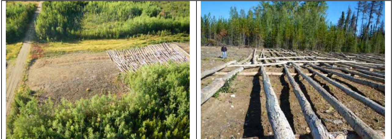
Figure 3 Example of Rollback Spread at a Road Intersection with a Pipeline ROW from the Air (left) and Ground (right)
