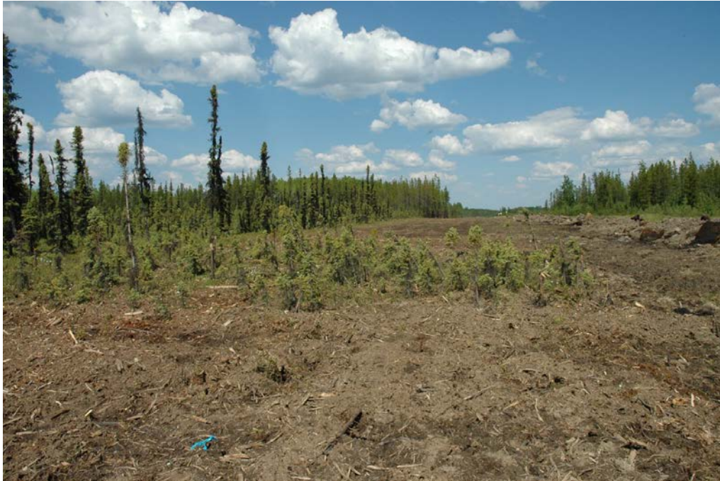
Plate 11: Example of a ramp-over area where a snow ramp was packed over vegetation in a treed lowland. The resultant vegetation screen will contribute to natural regeneration on the adjacent areas of the footprint. Site conditions and construction requirements can limit the use of this measure. Photo source: CH2M HILL.
