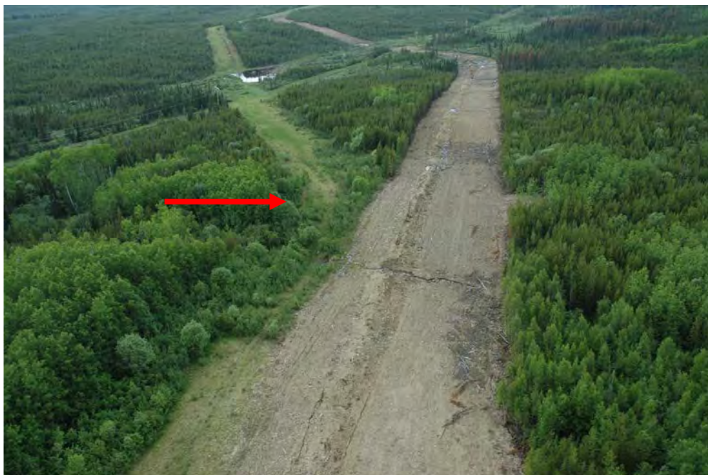
Plate 10: Example of a vegetation screen retained along edge of pipeline right-of-way at intersection with an existing linear disturbance. Vegetation screens block line-of-sight and can effectively manage access. Photo source: CH2M HILL.
