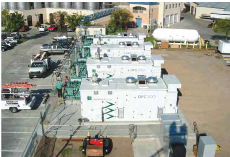
Figure 46: Fuel Cell installation at a brewery, 4 x 250 kW modules, from FuelCell Energy
