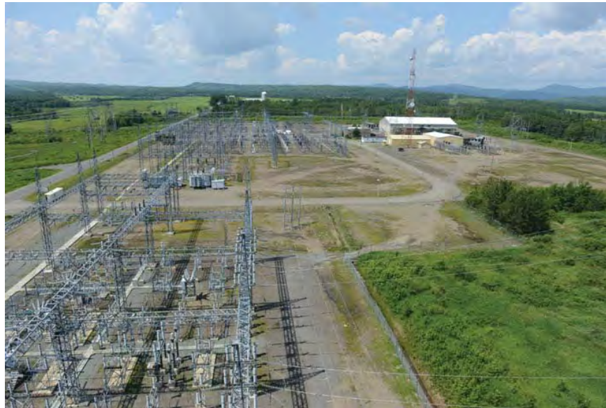
Figure 13: NB Power's Eel River HVDC Station
